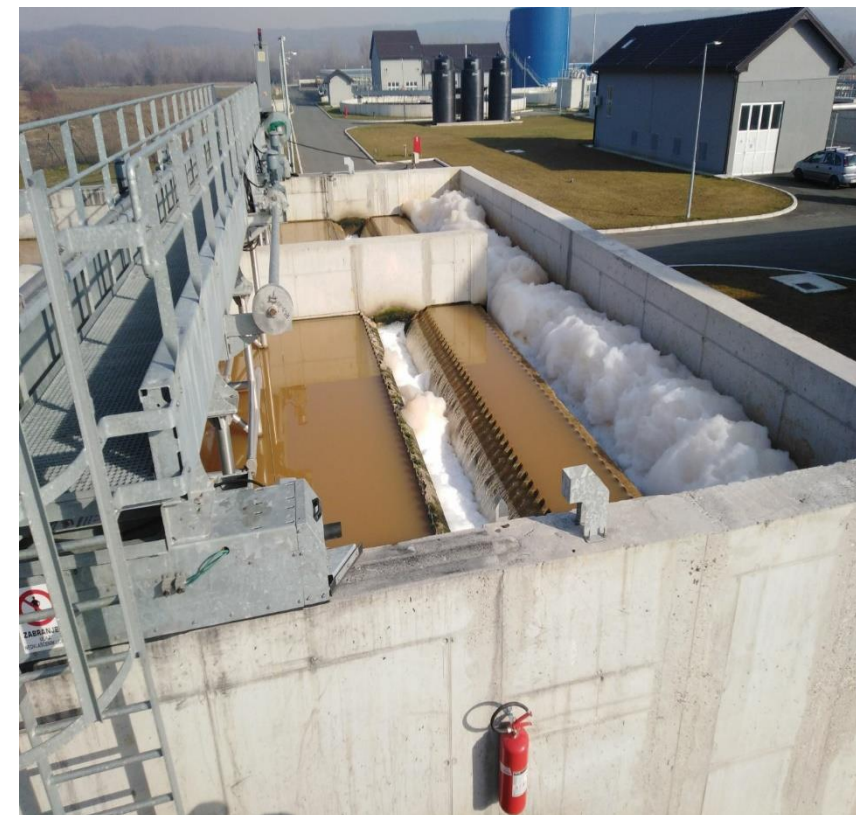
Appearance of foam and dark coloration in primary clarifiers
