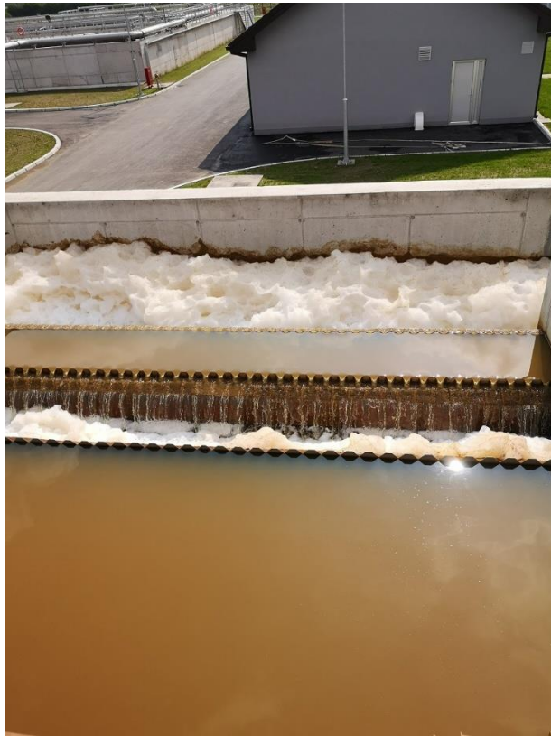
Appearance of the primary precipitator after the incident
