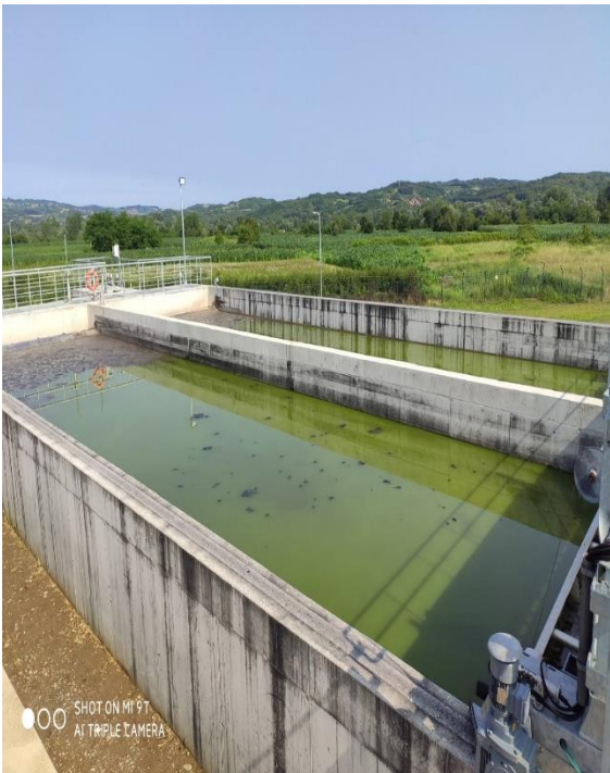
Appearance of green coloration in primary settling tanks
